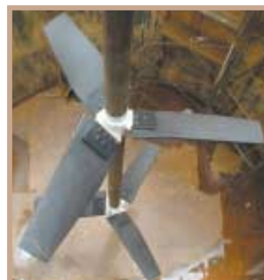
Agitator in CIL plant tank
