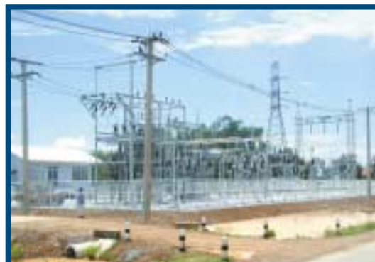
Completed company owned substation
